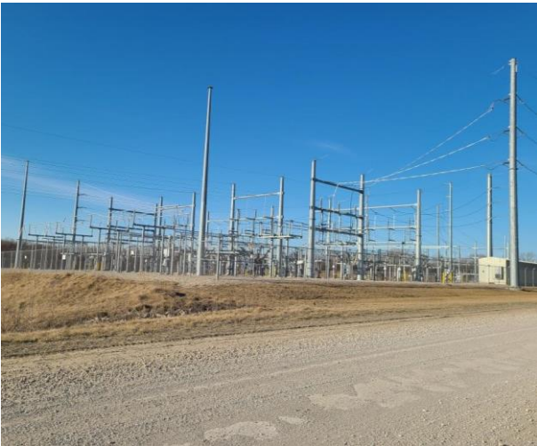
The Woody Substation on the east side of Ottumwa.
