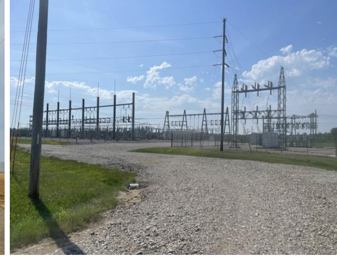
The Henry County Substation near Mount Pleasant.
