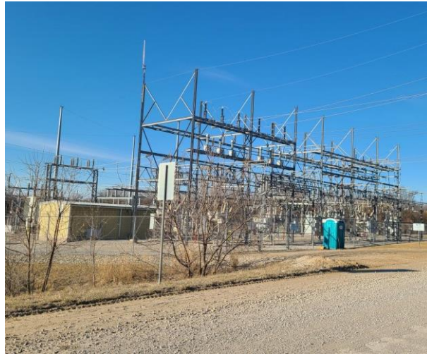
The Wapello County Substation on the east side of Ottumwa.
