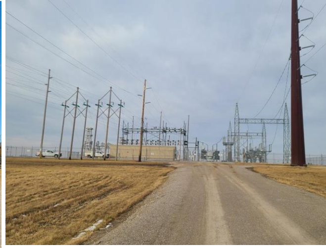
The Jefferson County Substation near Fairfield.
