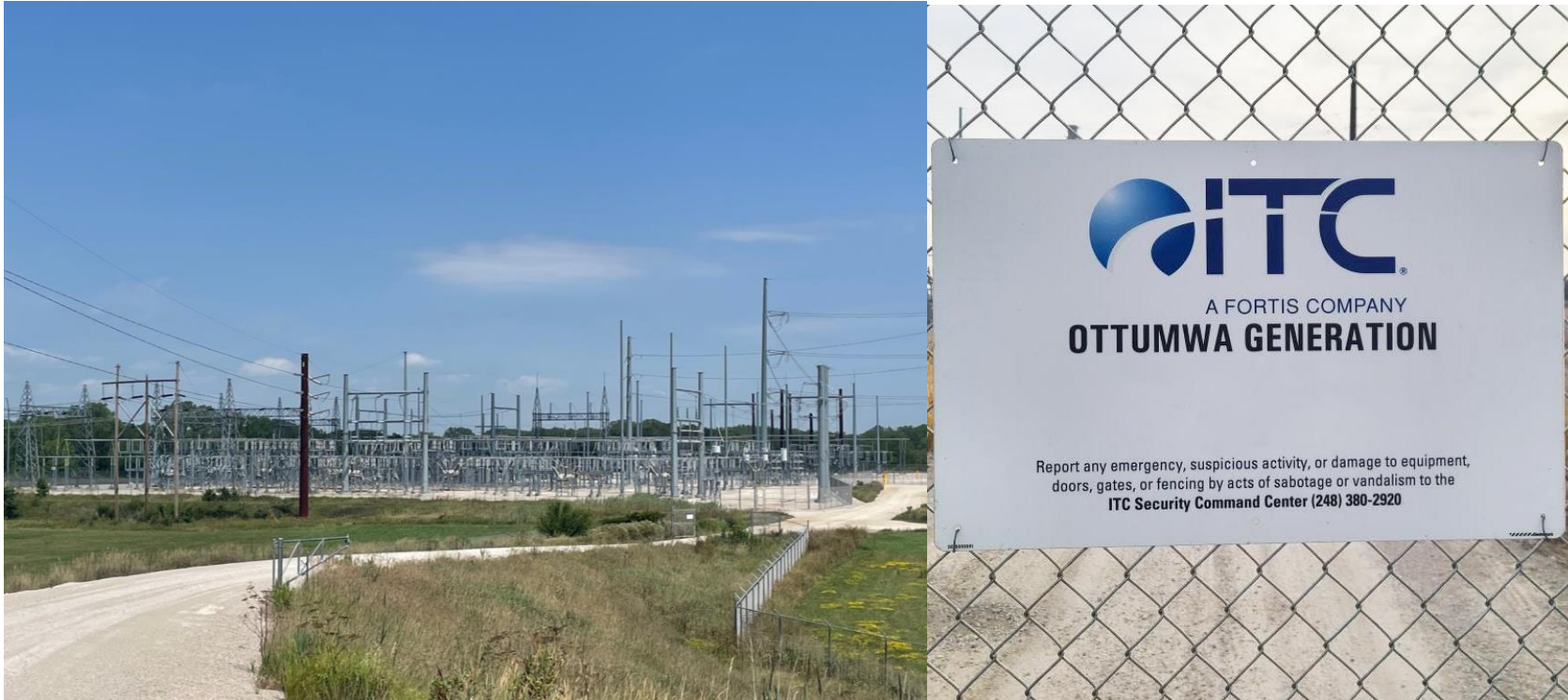
ITC Midwest's Ottumwa Generation Substation near Chillicothe, Iowa.
